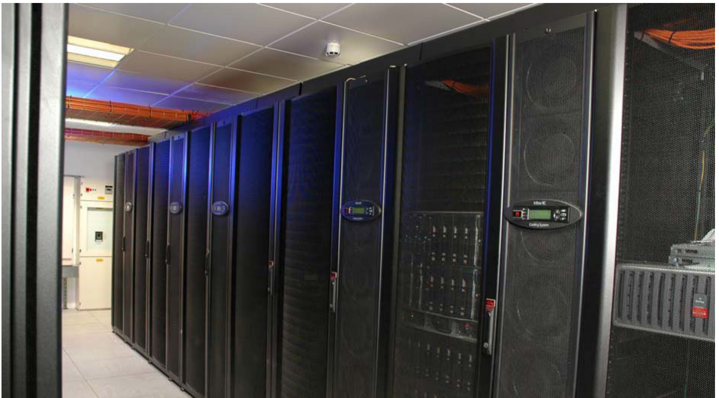
The completed cold aisle with just some of the shielded Net10G LSZH data cable in tray overhead
