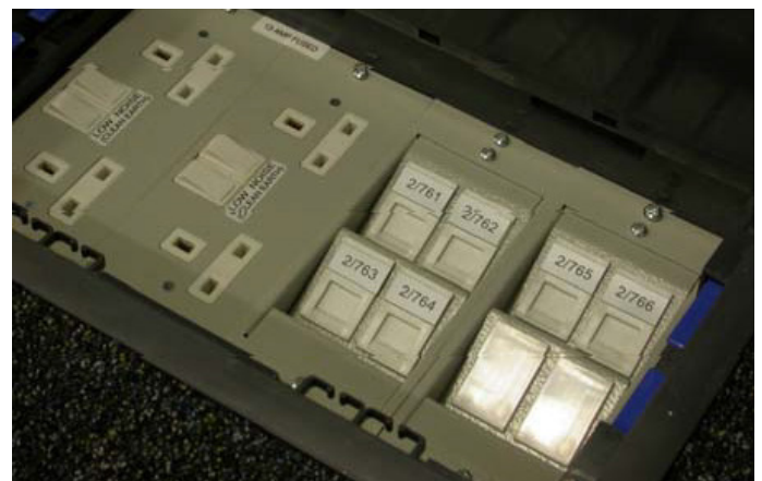
Floor box in one of the meeting rooms
