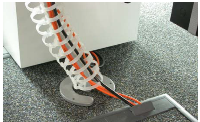
Cable management from each floor box to desk
