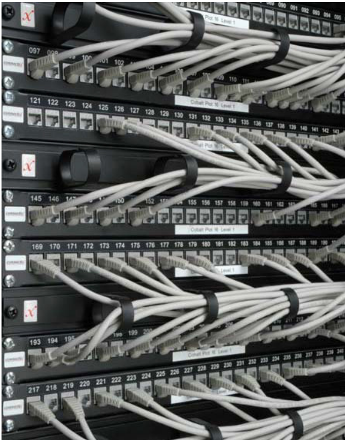
Net10G patch panels and cable management
