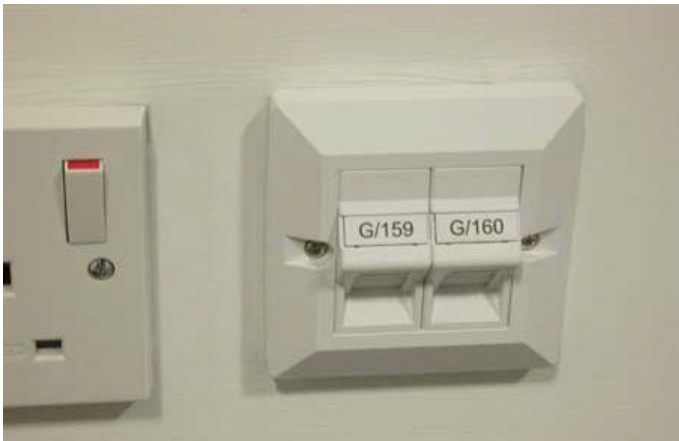
Angled wall outlets with Traffolyte labelling
